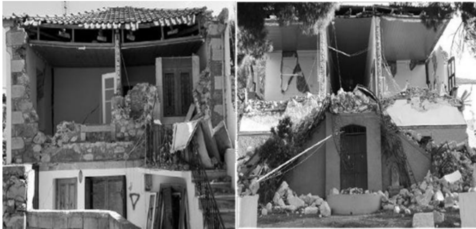
FIGURE 2.1: Seismic Damage in Conventional Masonry House Highlighting Failure at Wall Intersections (Cross-Junction Regions) [31].
