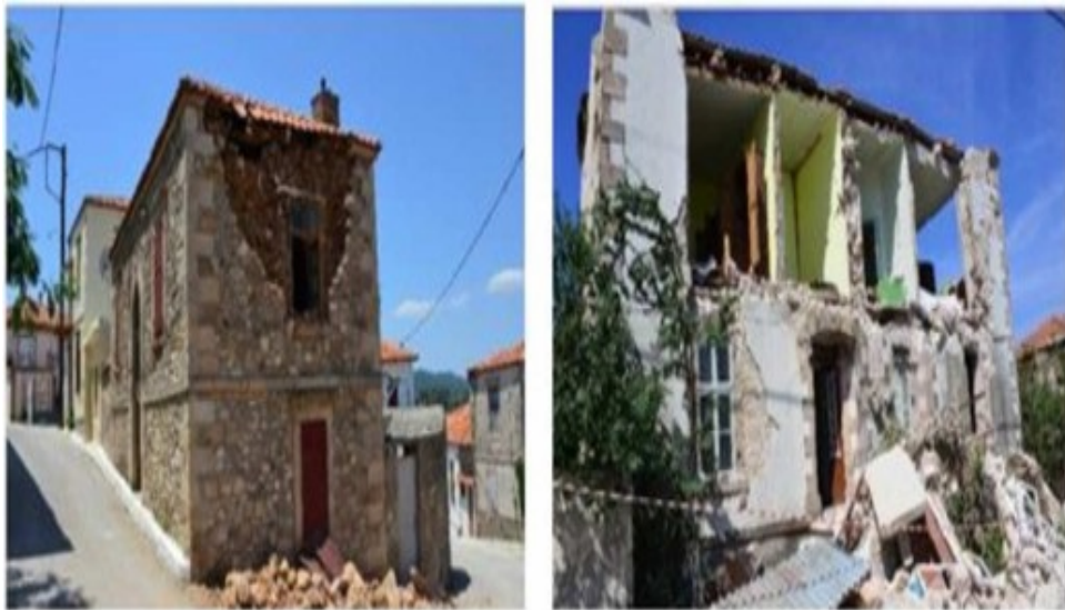
FIGURE 2.1: Damage to Masonry Buildings after Earthquake
