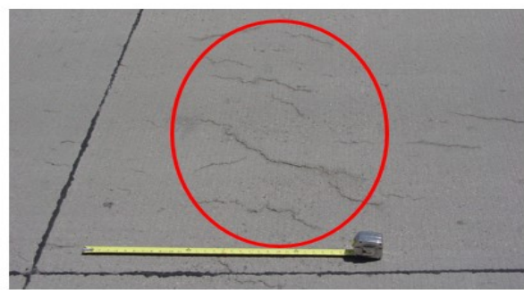
Plastic Shrinkage Cracking in Rigid Pavement
