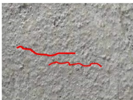
Early Age Micro-Cracking in Slab
