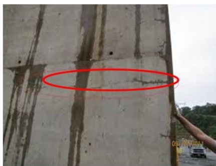
Cracks in Compression Member
