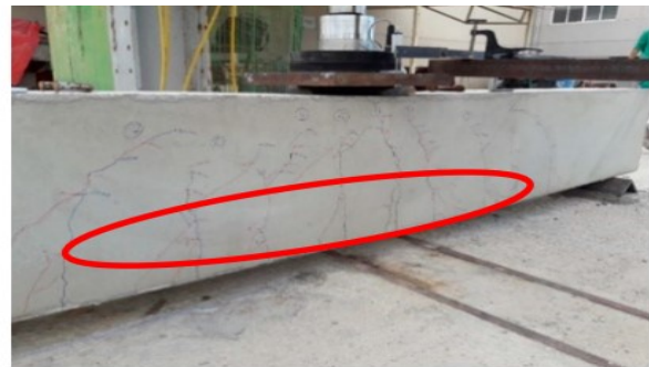
Cracks in Beams
