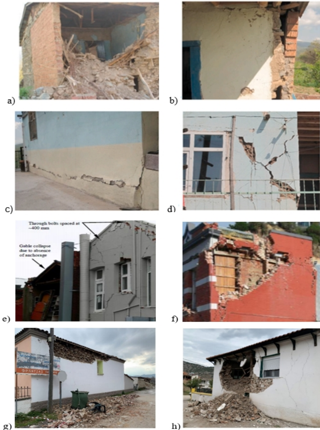
FIGURE 2.1: Failures in masonry structures: (a) and (b) out-of-plane damages, (c) and (d) in-plane damages [12], (e) and (f) out-of-plane separation [18, 19], (g) delamination and (h) out-of-plane failure [15].
