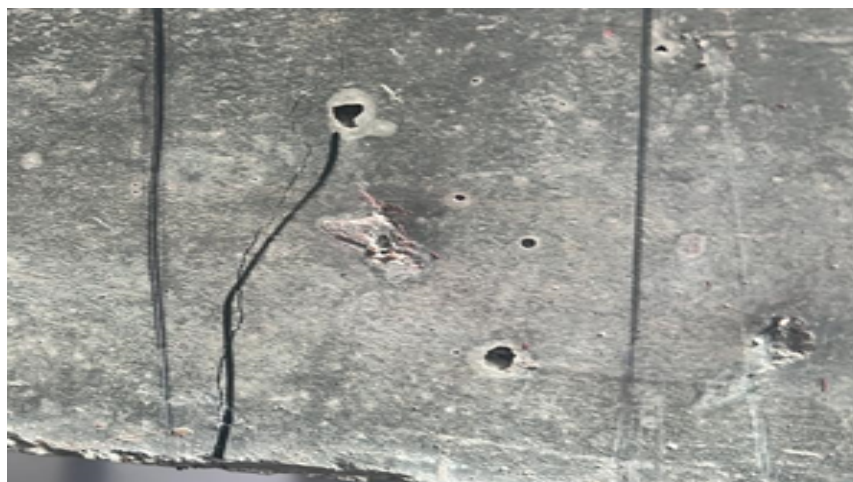
FIGURE 3.37: Vertical hair cracks
