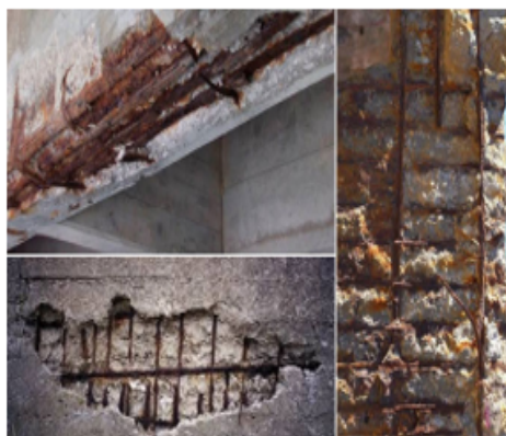
Fig c): Strength Deficiency due to Corrosion
