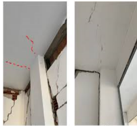
Fig b): Strength Deficiency due to earthquake cracks
