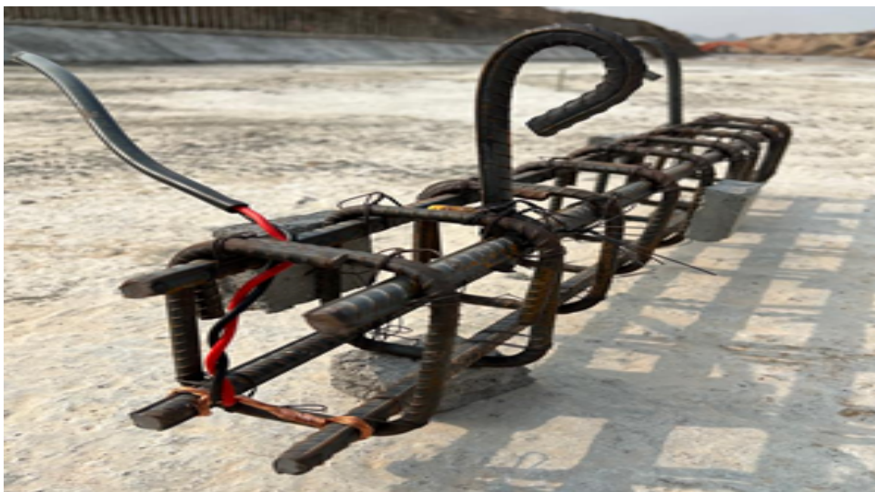
FIGURE 3.10: Lateral face of steel skeleton & electric cable connection
