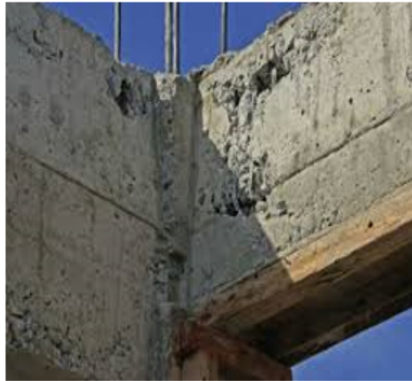
Fig a): Strength Deficiency due to poor workmanship
