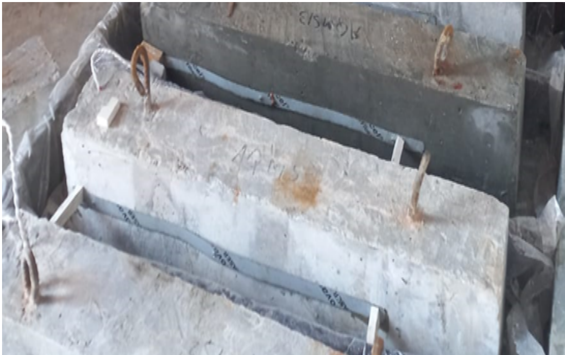
FIGURE 3.19: Stainless Steel cathode attached with beam
