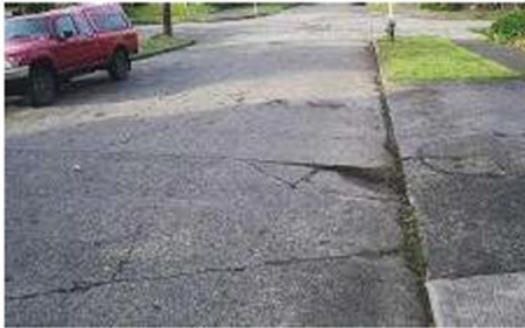
FIGURE 2.3: Corner Break on a Residential Street [13].
