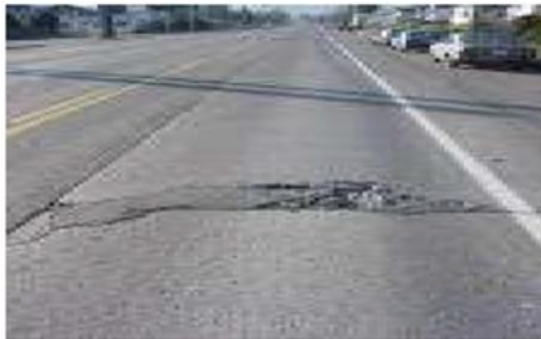
FIGURE 2.4: Spalling from a Bad Construction Joint [11].
